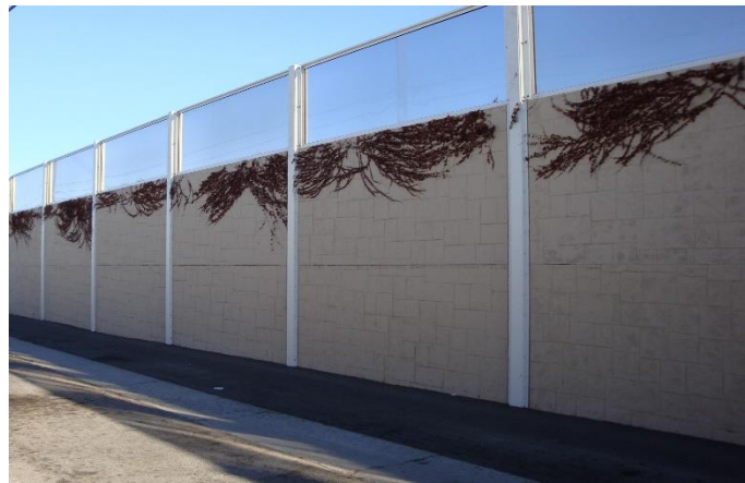
ACRYLITE® Soundstop Ready Fit System near Target on W Redondo Beach Blvd. in Gardena, CA
