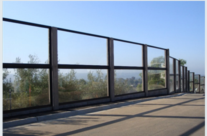
ACRYLITE® Soundstop Ready Fit System on Park Drive above the South Bay Freeway (CA-54) in Spring Valley, CA
