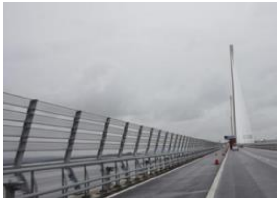
ACRYLITE® Soundstop Wind Barrier System with "C" shapes on the Queensferry Crossing Bridge in Scotland, UK
