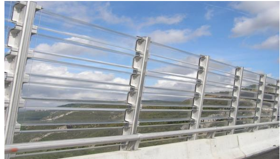
ACRYLITE® Soundstop Wind Barrier System with "C" shapes on the Crni Kal viaduct in Slovenia
