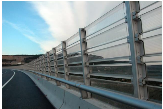
ACRYLITE® Soundstop Wind Barrier System with "C" shape design using colorless Soundstop GS CC on the Crni Kal viaduct in Slovenia
