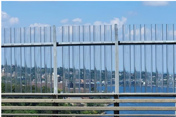
ACRYLITE® Soundstop Wind Barrier System with “C” shapes on the Verrazano Bridge in New York City
